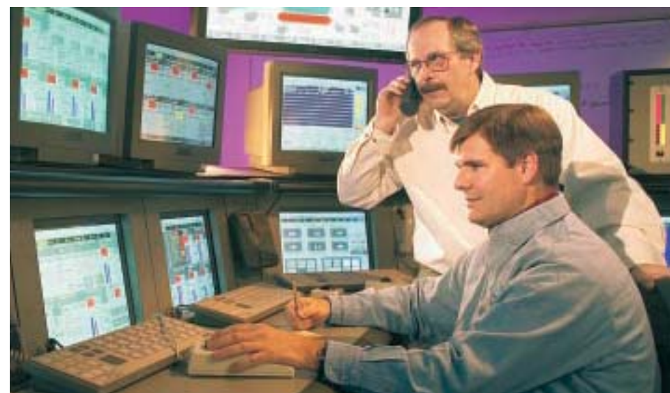
Robin Dahline, sitting, and Denny Johnson in the new control room at Minnesota Power's largest generation station, the Boswell Energy Center in Cohasset, Minnesota.
